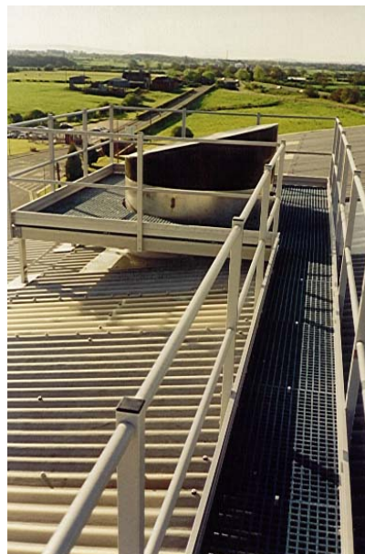
Typical access walkway in rooftop location. Low weight reduces loads on roof support structure. GRP materials resisted all weather conditions in this exposed situation.
